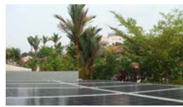
#2 PROJECT CLOSED RESIDENTIAL SOLAR PV @ TERANG BULAN AVE (5.5KWP)
